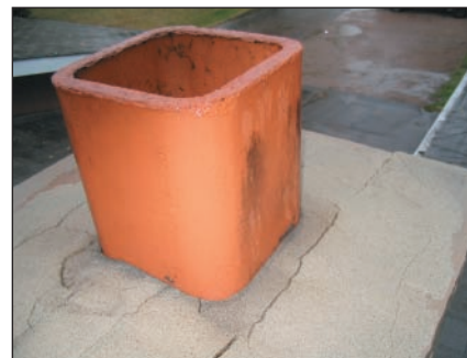
Damaged crown and eroded mortar joints should be repaired before relining.
