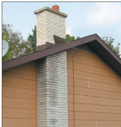
Stains like these are caused by condensation of moisture and creosote from cool flue gases.
